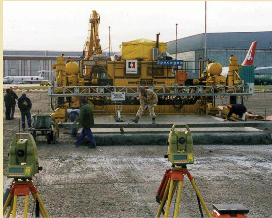
Above: belt and braces - two robotic total stations provide control for a paving machine laying concrete while the airport is open for business as usual.
