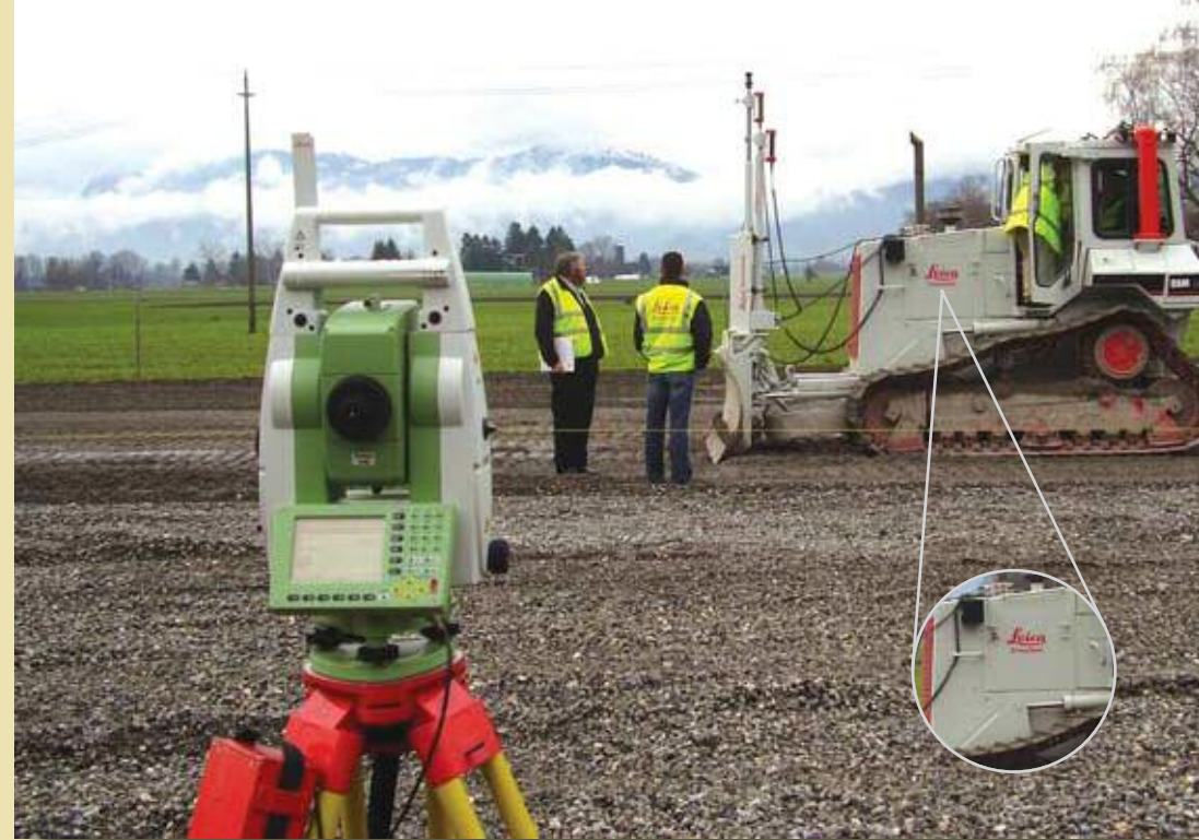
Above: a TPS1200 total station tracks the prism and communicates with the computer on the bulldozer to keep it on line and level. Meanwhile, is this the first of a line of Leica bulldozers?
