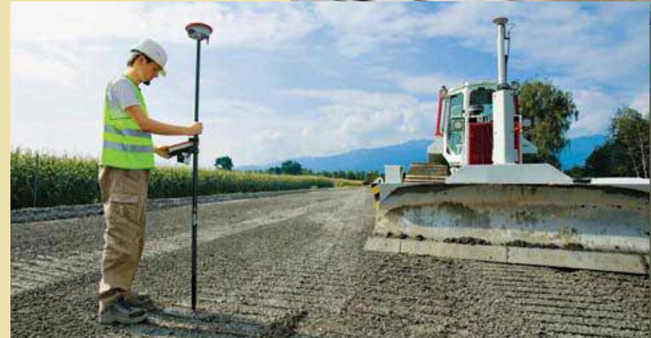
Above: a surveyor captures a position and sends it to the bulldozer so it can commence work.
